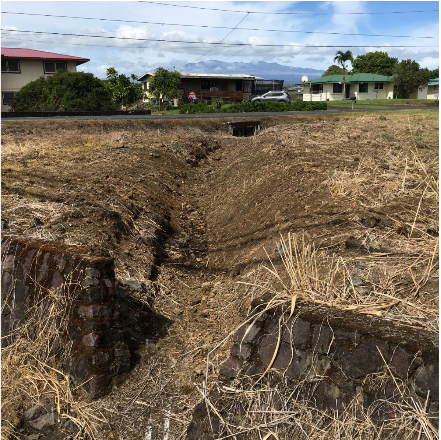
Unconfined drainage ditch at Southwest corner of property
